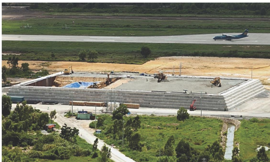
The treatment structure being loaded with contaminated soil and sediment and covered by a gravel plenum layer in Fall 2013 (Photo credit: TetraTech, Inc.)
