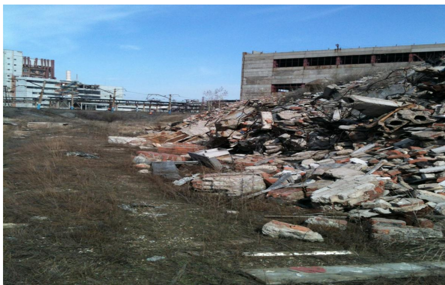
Fig. 1. Storing of building breakage of destroyed buildings, Ufa, Khimprom, 2013
