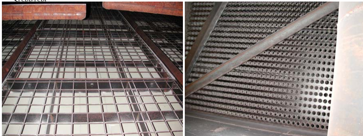
Picture 15, 16: 4 stage catalyst box without dust precipitations give very low I-TEQ PCDD/PCDF of 0,001 \text{ng}/\text{m}^3
