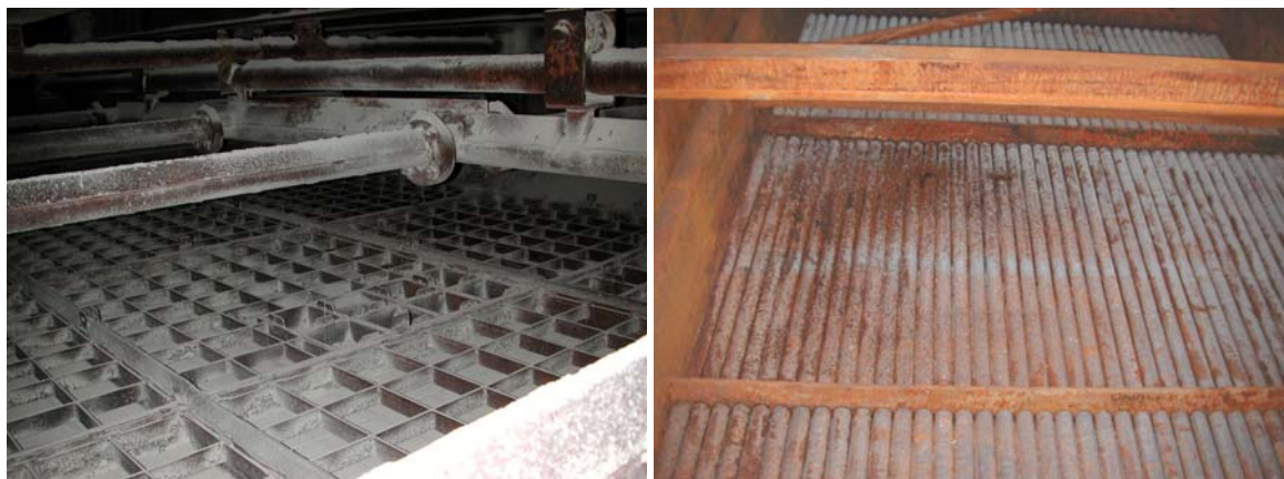
Picture 17, 18: Catalyst box with dust precipitations 2 years before with I-TEQ PCDD/PCDF of 0,03 ng/m 3
