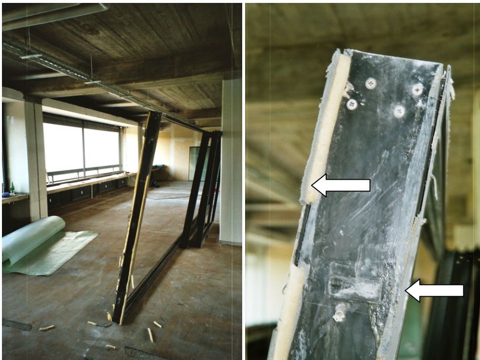
Figure 2: Window frame, rabbet with elastic joint seal containing PCB
