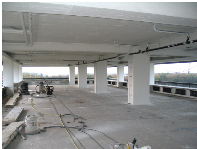
Figure 3: View of a floor after second remediation
