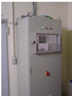
Figure 1: AMESA control cabinet
